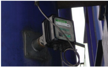
Carbon Black Filter Plant with Electrodynamic Sensors
